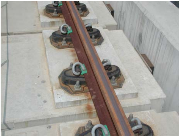
Figure 11 Close-up view of KCRC viaduct floating slabs with low stiffness rail fasteners
